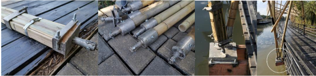
Figure 5. (Two in Left) Images also show nozzles for culms and bamboo splits after being installed, and (Two in Right) Connectors were fabricated in real construction.
